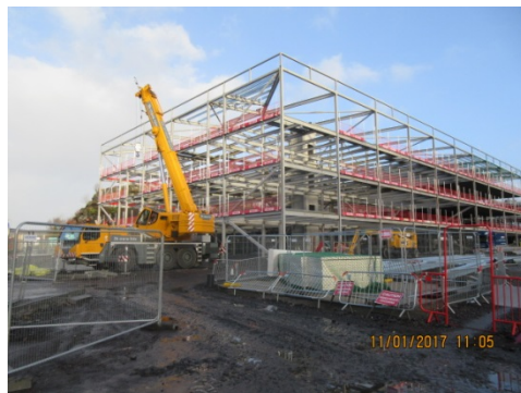
Photograph 1 – The gable end of the new school building behind McCall Terrace. This marks the completion of the structural steelwork.
